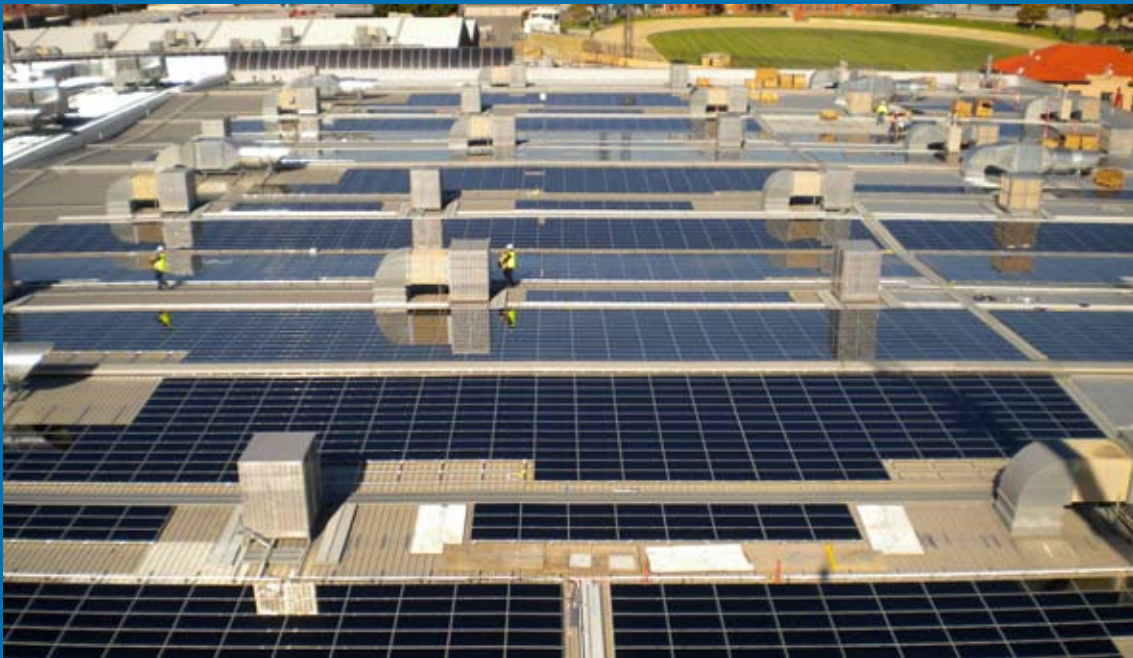
Australia's largest grid connected solar power system at the Adelaide Showground
